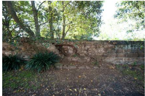
Figure 192: Wall along road south-west of house to car parking area showing damage to stonework. Paul Davies 2014.
