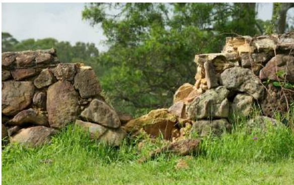
Figure 168: Stone wall along driveway, 1980s, looking south showing an area of recent damage (since repaired). Paul Davies 2013.
