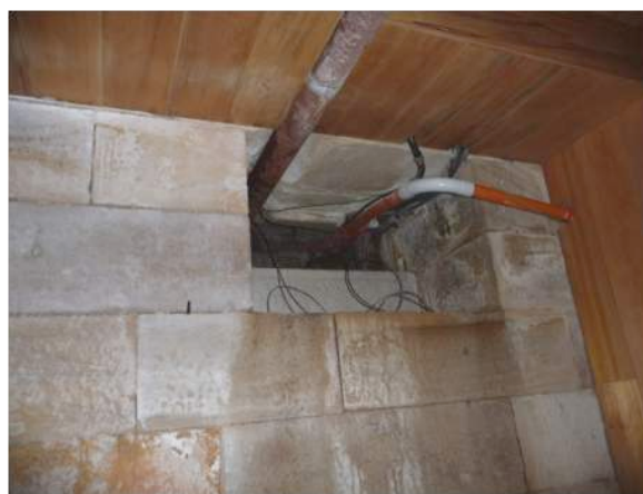
Figure 297: Partly bricked up vent and intrusive services on northern wall in Basement room B10; also shows evidence of salt attack and spalling on the original sandstone walls
